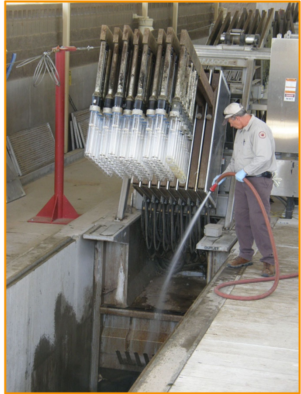
FIGURE 52. CAVE CREEK WATER RECLAMATION PLANT, CITY OF PHOENIX
