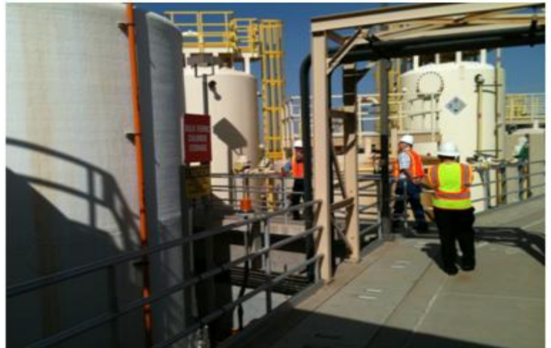
24 th Street Water Treatment Plant Chemical Storage Area
